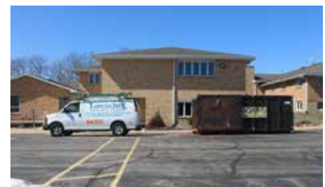
The south entrance is a construction entrance and will soon be the site of exterior construction.
